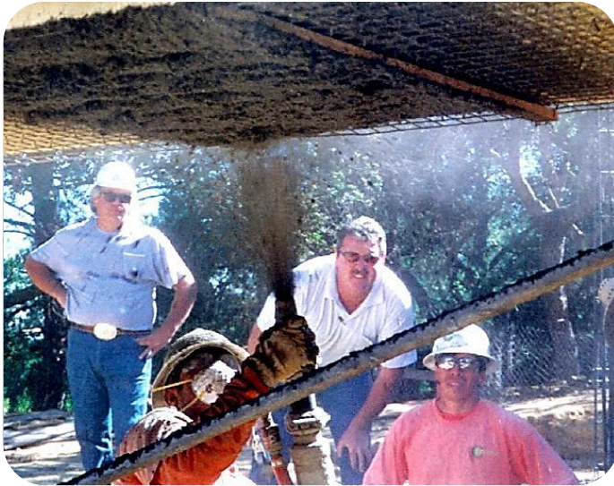
Vertical shotcrete spray has no rebound with immediate adhesion to the ceiling.
